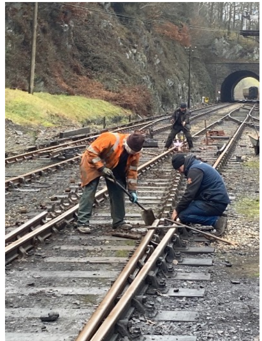
Photo (left) shows close up of one of the new nose and wing rail sections.
